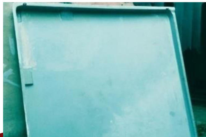
FRP Trough Below AC Unit
